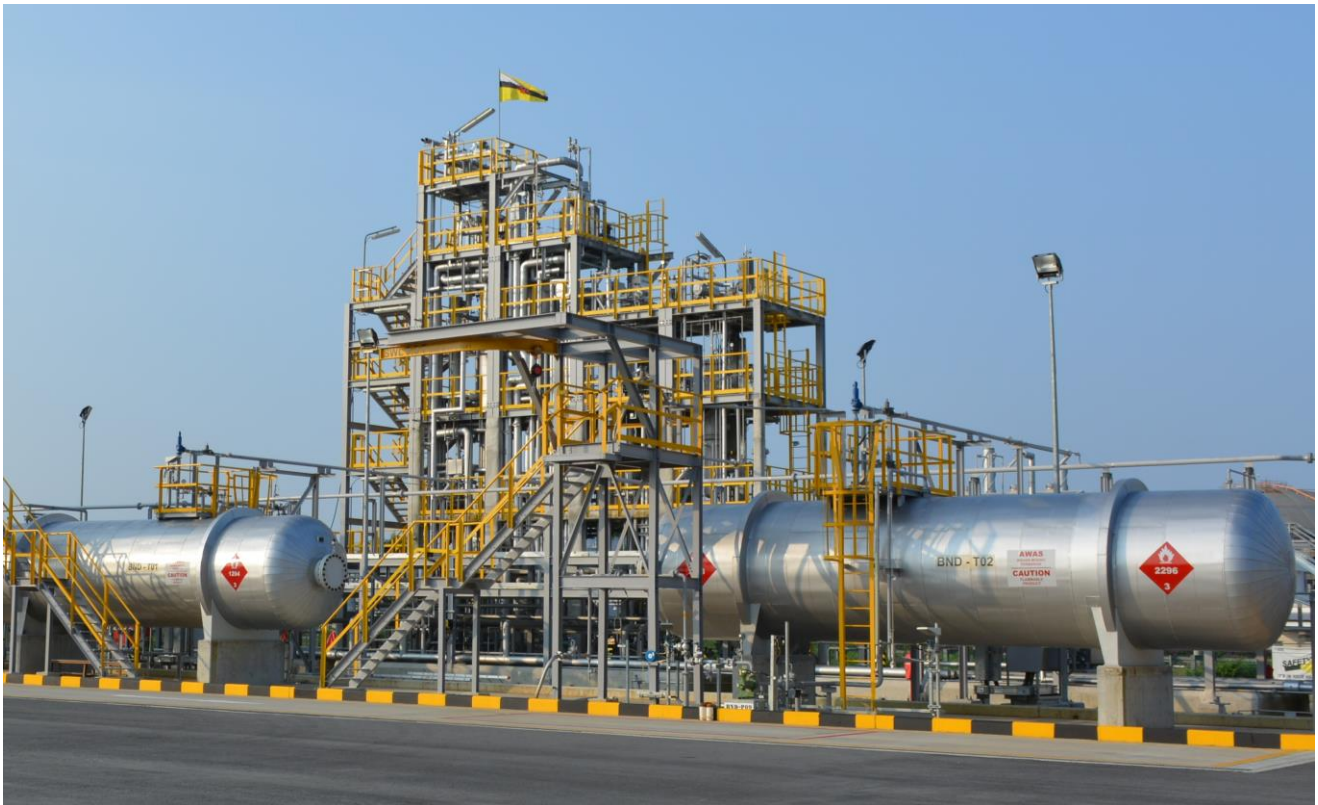
Hydrogenation plant in Brunei
