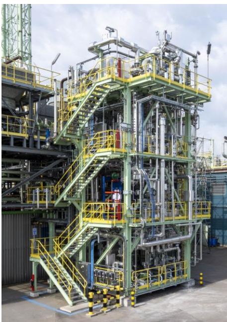
Qpinch unit in port of Antwerp, Belgium. Photo: ©2021 Borealis.
