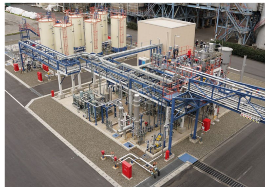
Kawasaki Dehydrogenation Plant
