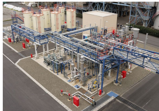
Kawasaki Dehydrogenation Plant
