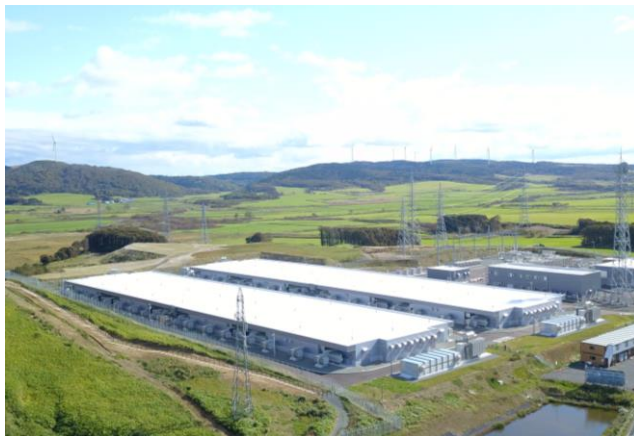
Battery Energy Storage System
