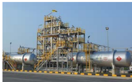
Hydrogenation plant in Brunei Darussalam
