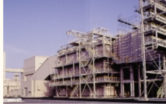
Chiyoda completed construction of the one-million-kilowatt Haramachi thermal power station no. 2 unit for Tohoku Electric Power Co., Inc. The Company constructed and installed Chiyoda Thoroughbred 121 flue gas desulfurization units, gas-gas heaters, and desulfurization fans.
