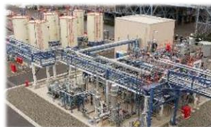
Dehydrogenation plant in Keihin Refinery, TOA Oil*3
