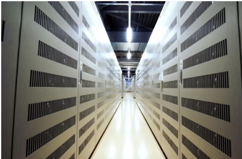
Energy Storage System
