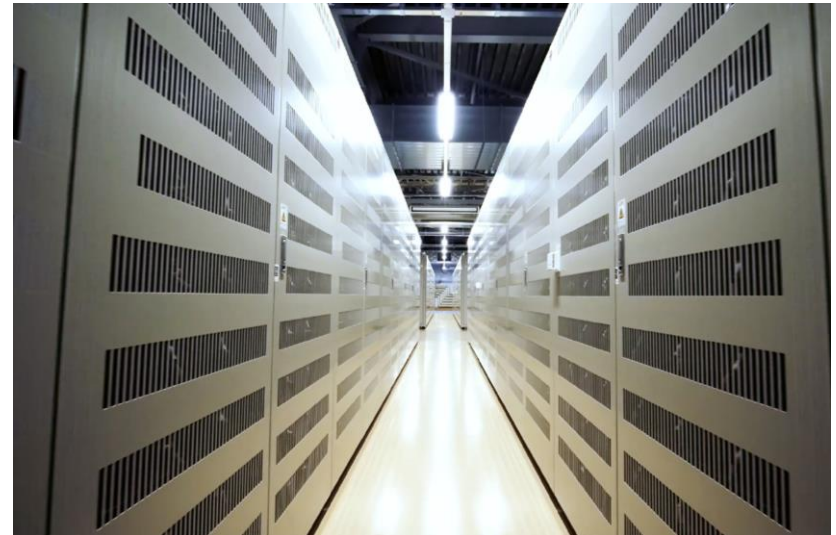
Energy Storage System
