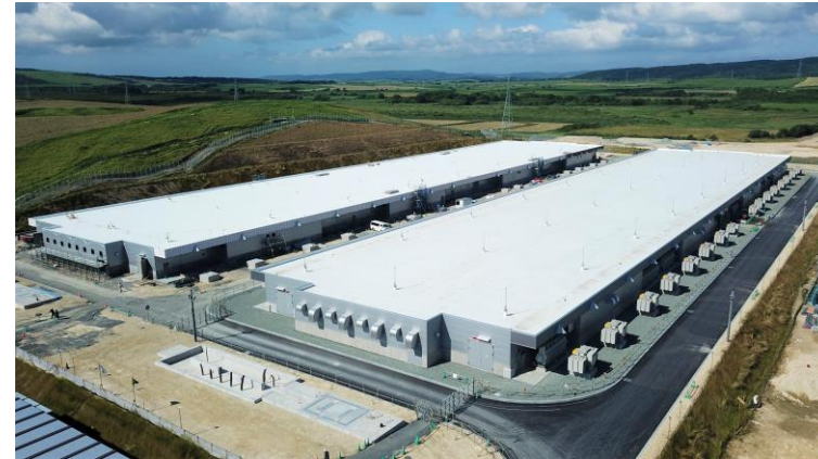
North Hokkaido Wind Energy Transmission Corporation. Battery Energy Storage System Construction Site (Photo as of July 2020)
