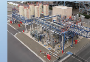
Dehydrogenation Plant at Kawasaki Waterfront
