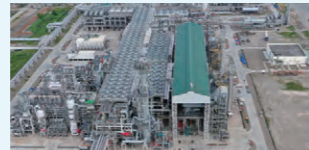
Liquefied natural gas plant for BP Berau
