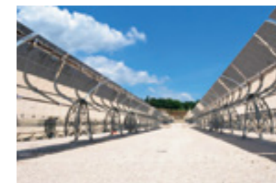
MSPT-CSP (Molten Salt Parabolic Trough Concentrated Solar Power) Demonstration Plant
