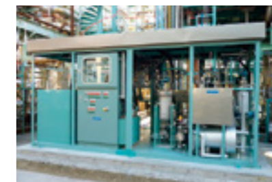
Test equipment installed at the Kawasaki Plant of JX Nippon Oil & Energy Corporation
