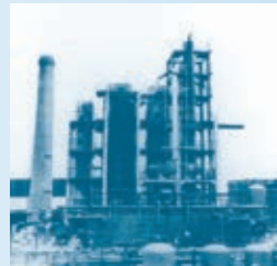
Construction to rebuild the Kawasaki refinery of Mitsubishi Oil Co., Ltd. (present JXTG Energy)
