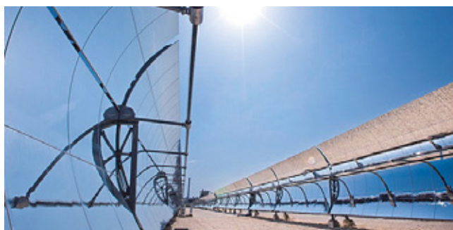
Solar concentrating system of pilot plant in Sicily, Italy
