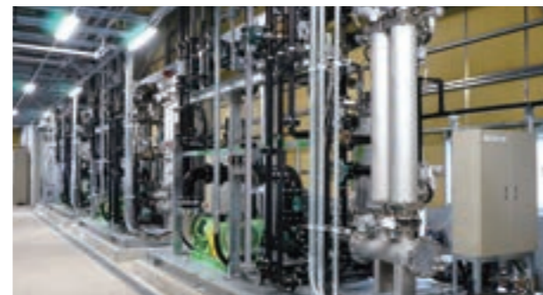
Yabase oil field produced-water treatment demonstration plant
