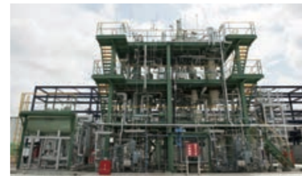
Pilot plant demonstrates SPERA hydrogen system
